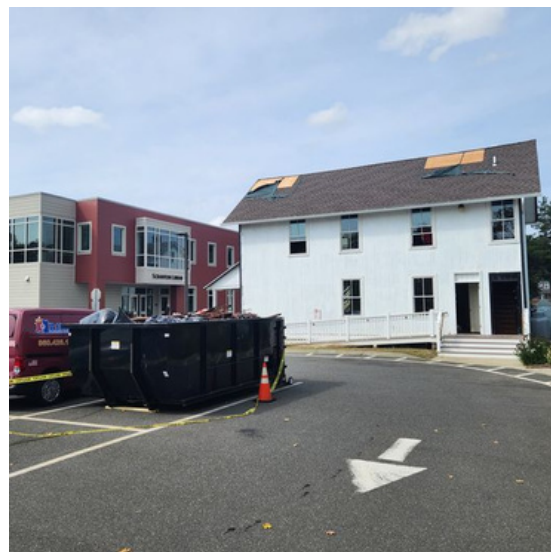
20 Wall Street begins reconstruction after a fire damaged the building in early 2023.
